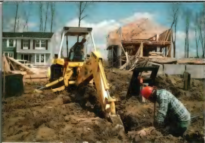
Workers prepare to lay cable in a sold-out town-house development in Columbia, Md.
